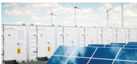
Battery energy storage systems (BESS)
